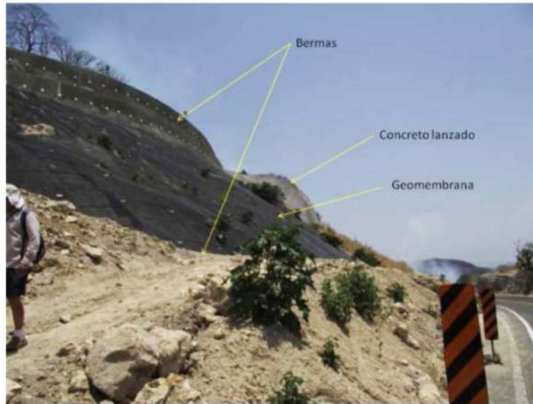
Image 4 Case 1. Ocozocoutla-Arriaga motorway (190 D) (Photo 1). Location: km 25 (16 ° 41'54.36 "N, 93 ° 32'32.56" W). (Photo 1). The zone corresponds to the contact of two units: Tritic-Jurassic shale-sandstone and lower Cretaceous limestone-shale.
