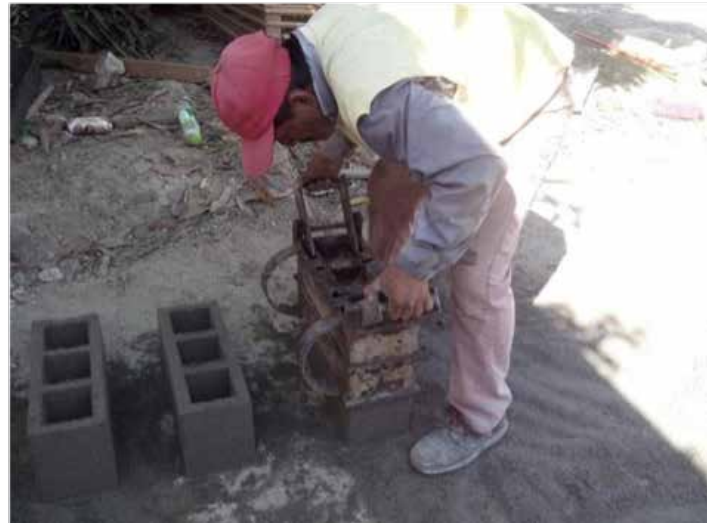
Image 17. Mold Removal Process. Source: Own elaboration
