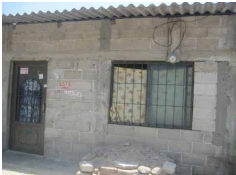
Image 7. Absence of vertical reinforcement in openings. Source: Own elaboration
