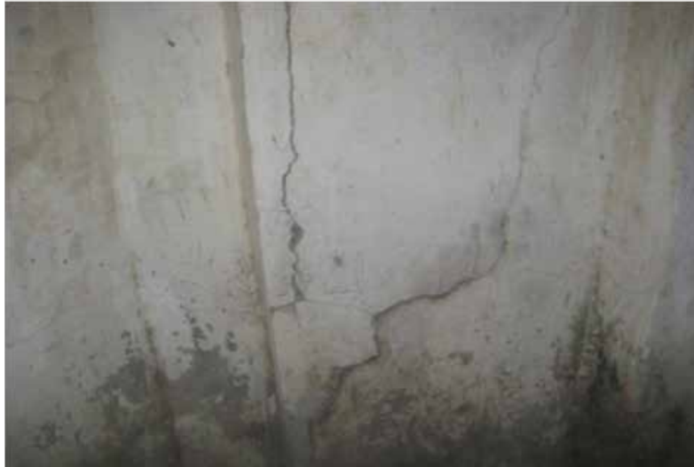
Image 6. Cracks at the intersection of walls
