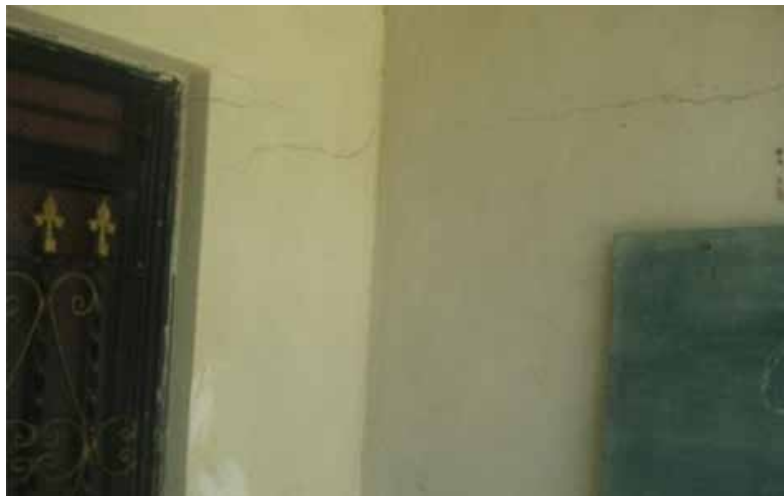
Image 5. Cracks at the intersection of walls
