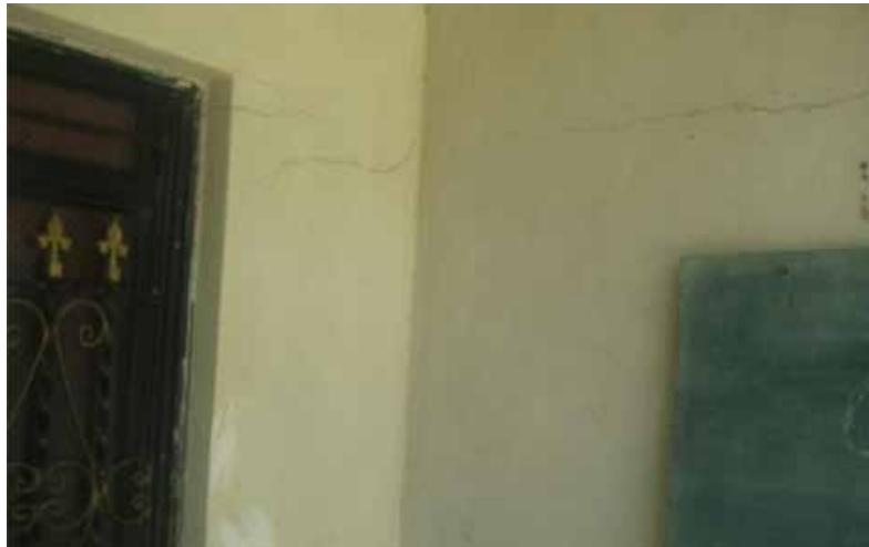
Image 5. Cracks at the intersection of walls
