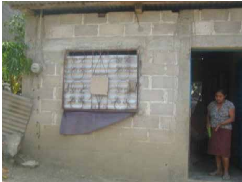
Image 8. Absence of horizontal reinforcement in window. Source: Own elaboration
