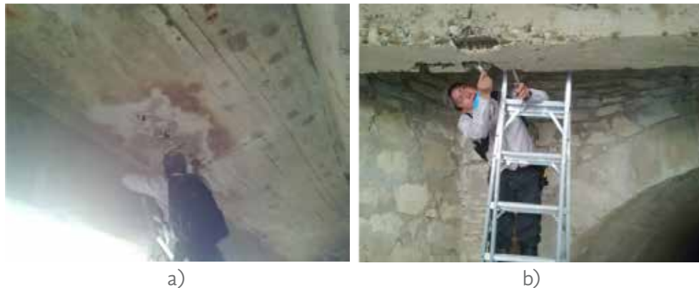
Figure 14. a). Measurement of deterioration (segregations) in slab and b). Measurement of beam's segregations with digital vernier "Mitutoyo" and transparent millimetric ruler
