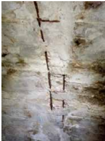
Figure 12. Underground culverts-arch's internal lining with strong steel corrosion problems and crystallized salts from concrete leaching (Mundo, 2019)
