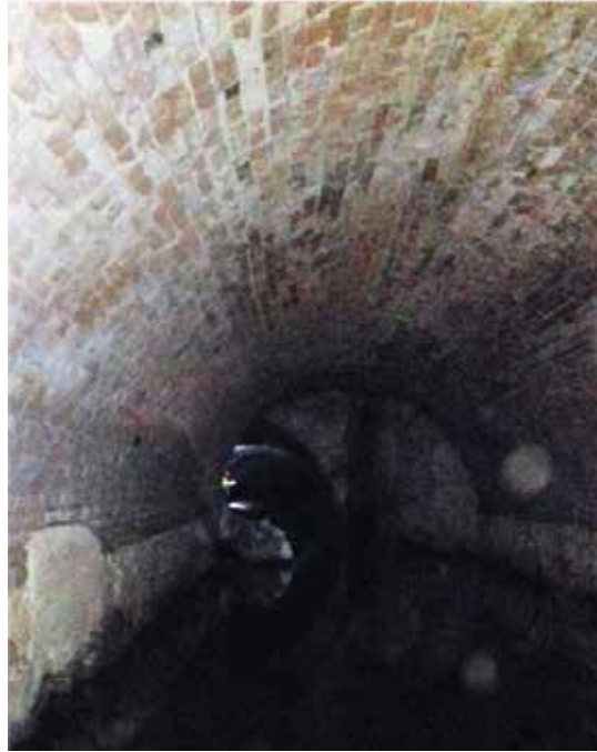
Figure 8. Brick underground culverts-arch's general view with efflorescence presence (Mundo, 2019)
