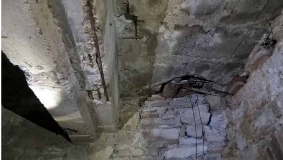
Figure 6. General view of slabs and beams with various pathologies
