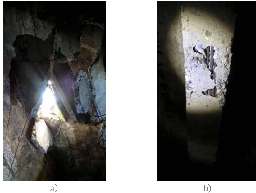
Figure 5. a). Slab collapse and b). Areas without concrete cover and with visible concrete segregation in beams of the RC structure
