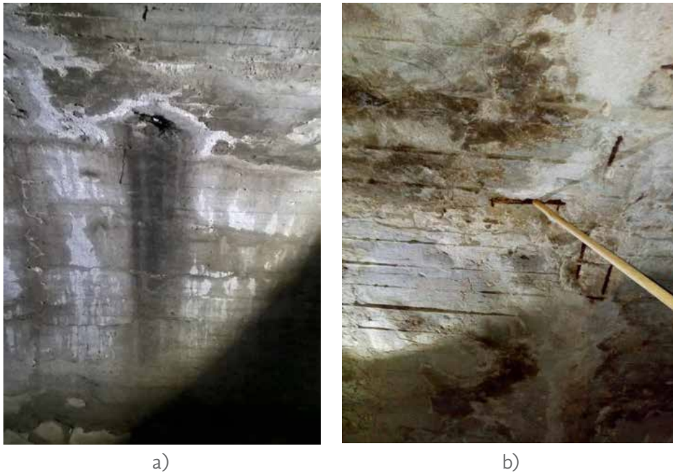
Figure 3. Material degradation of the “San Roque underground culverts-arch” structure (Mundo, 2019)
