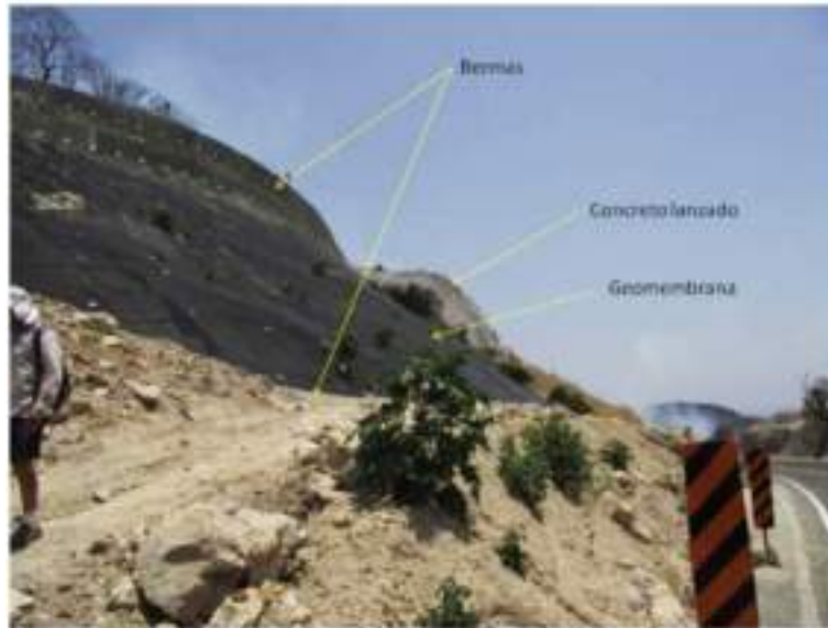
Image 4 Case 1. Ocozocoutla-Arriaga motorway (190 D) (Photo 1). Location: km 25 (16 ° 41'54.36 "N, 93 ° 32'32.56" W). (Photo 1). The zone corresponds to the contact of two units: Tritic-Jurassic shale-sandstone and lower Cretaceous limestone-shale.
