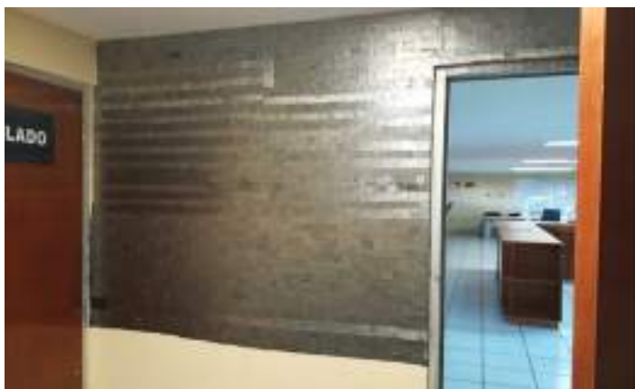
Image 3. Wall being lined with lead sheets, a contaminating radiographic waste material
