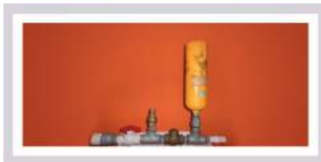
Foto 5. Hydraulic ram pump, Research Center, School of Engineering
